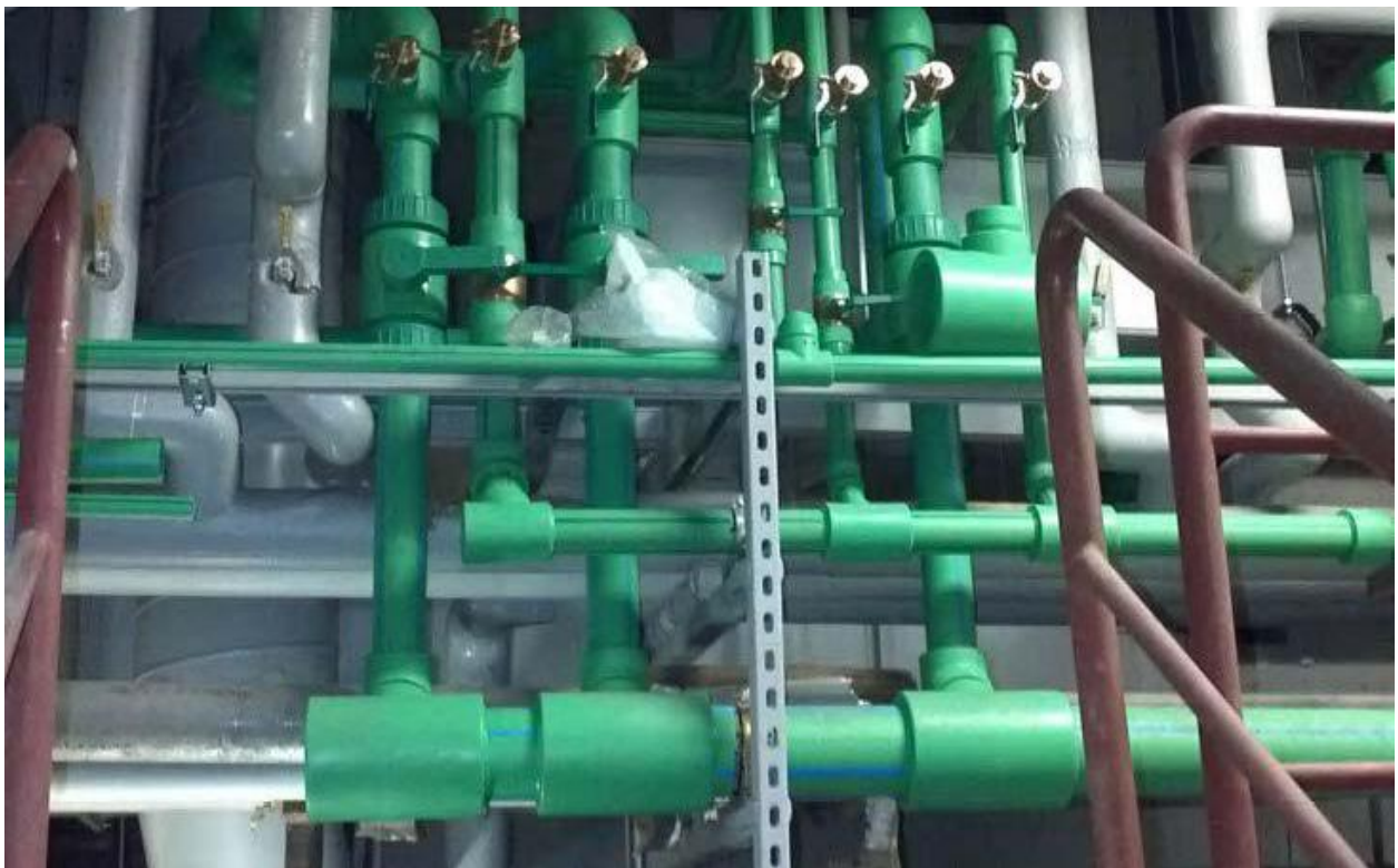
Pumping System for Supply Water
