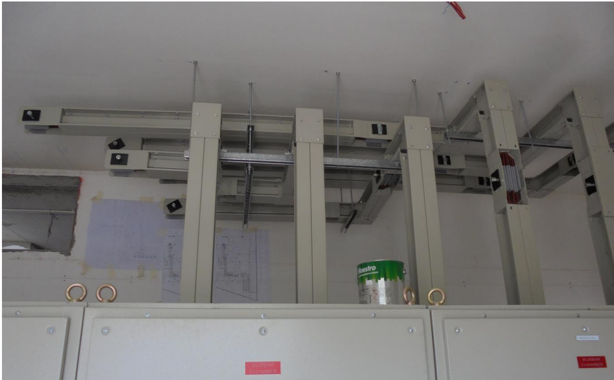
BUS BAR Riser & TOP OFF Unit
