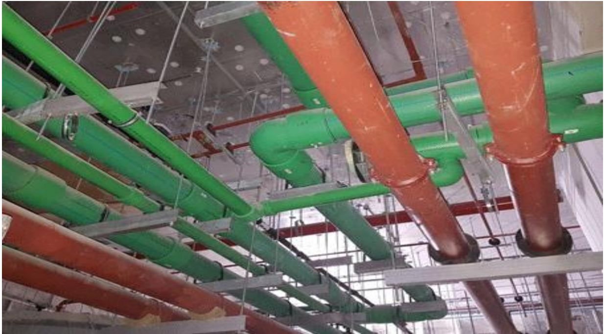
PPR Piping for Supply Water
